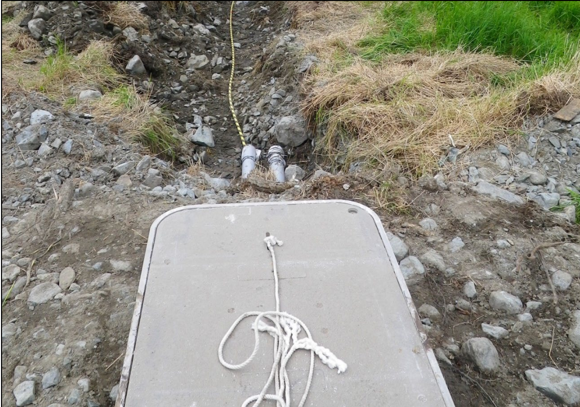
Photograph 2: Typical Beach Manhole with Conduit Stubs and Pull Rope
