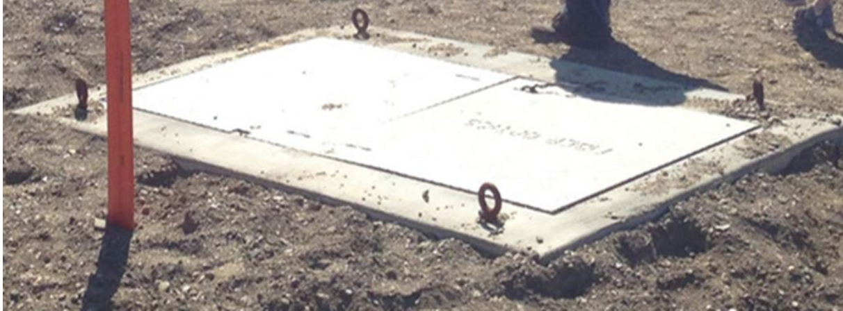
Figure 5. Typical beach manhole.
