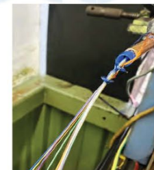
Closeup of 24 Fibers
