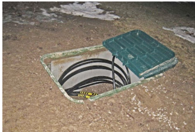
Figure 25: Cable Vault with extra FOC cable
