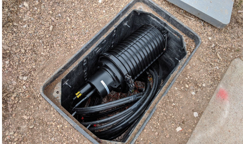
Figure 24: Handhole with FOC and splice case
